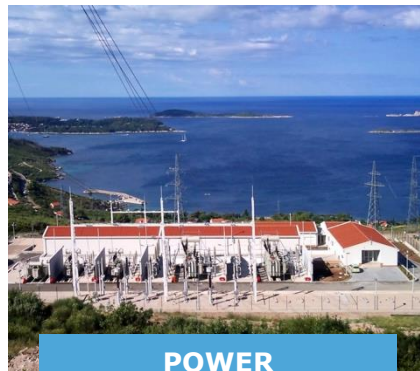
POWER TRANSMISSION AND DISTRIBUTION
