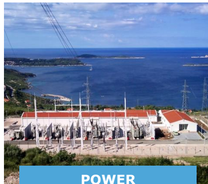
POWER TRANSMISSION AND DISTRIBUTION
