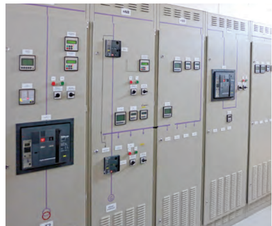
Industrial LV power distribution cabinet for industrial plant
