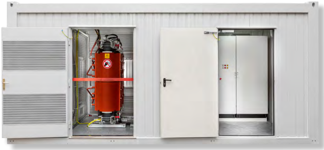
KonSol – converter equipment in a container at a PVPP project in Croatia
